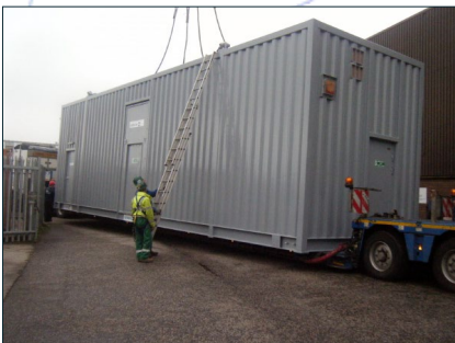
Load out of the modules from the UK to Belgium topsides Fab yard
